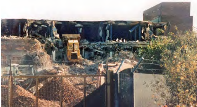
Demolition of the Loughborough cold store converted to RGHQ 3.2, showing internal structural detail. Photo Keith Ward
